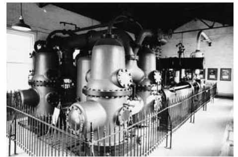
Crystal Spring Pump Station Photograph Courtesy of VDHR
