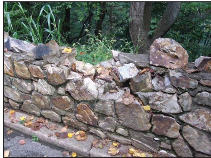
Deteriorating rubble walls. Photograph courtesy of Nancy Dye.
